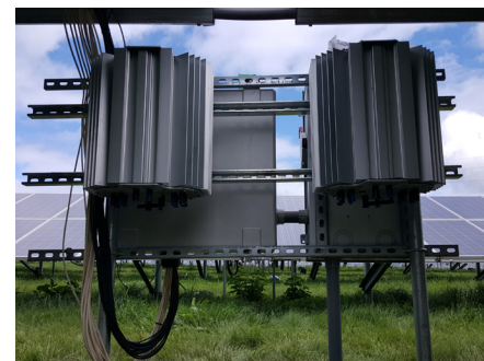
Alencon's power electronics hardware installed at a solar array. (Photo courtesy of Alencon)
