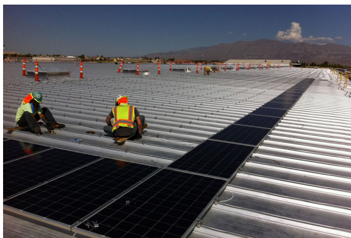
Solar installers work on the rooftop of a 110,000-square-foot Republic Services building in North Las Vegas. (Photo courtesy of Bombard)
